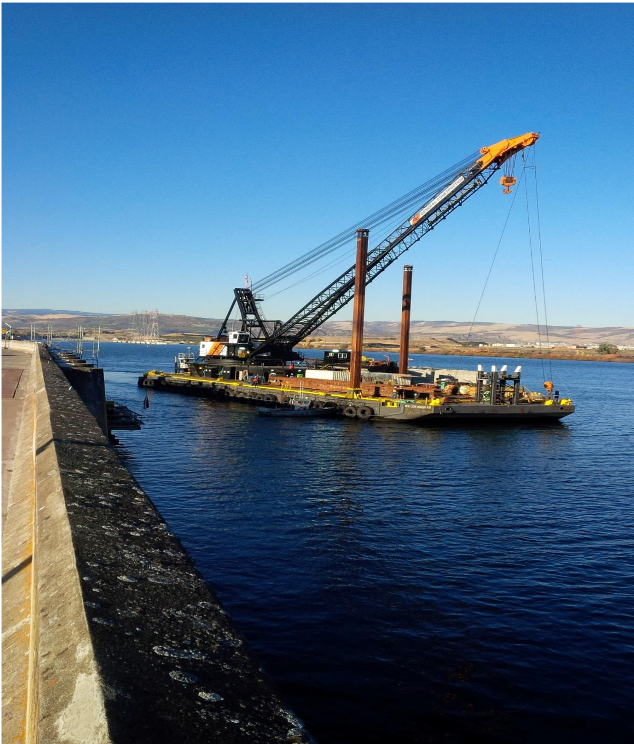
Barge crane setting up for AWS forebay work near east fishway exit.
